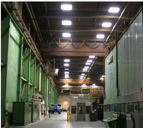
Energy-efficient lighting at Madison Paper
