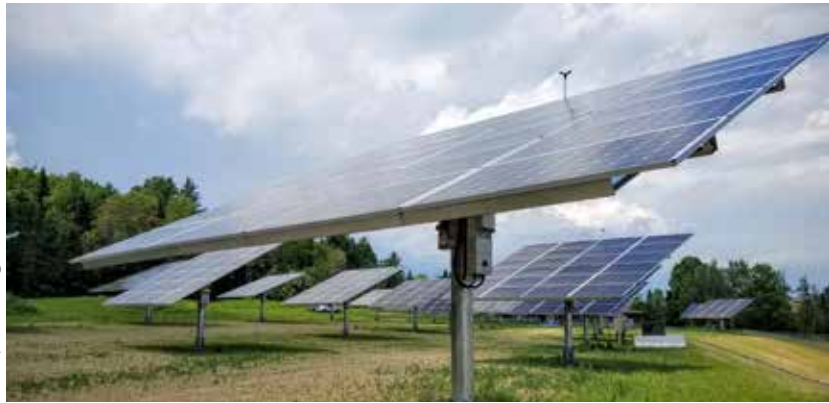
Solar panels in Aroostook County
