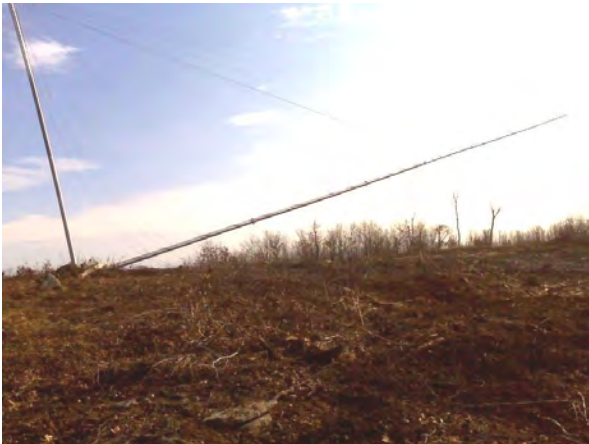
The meteorological tower on Saddleback Mountain was laid on its side and tilted upright when it was first installed.
