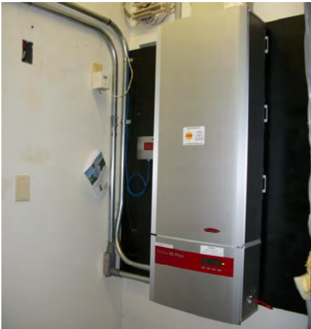
Inverter Room: Excellent Condition
