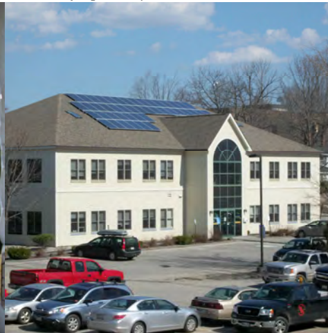
Rooftop Array: Excellent Condition
