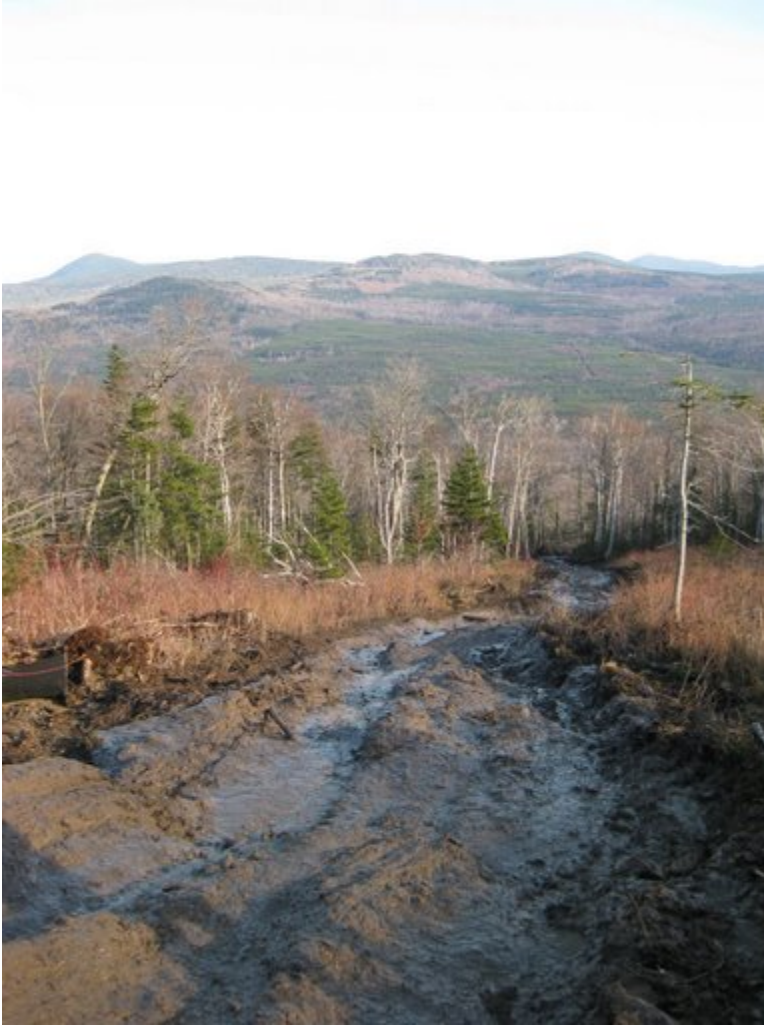
Heavy mucked wheel ruts along the skidder access road overlook A18 site preparation in the background.
