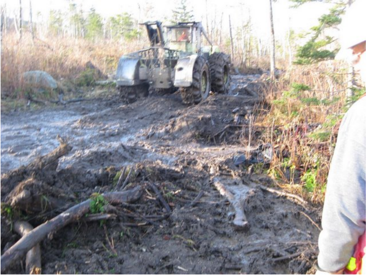
Skidder in mud: A short 6' section of silt fence could not hold back the volume of sedimentation that ran down the wheel ruts.
