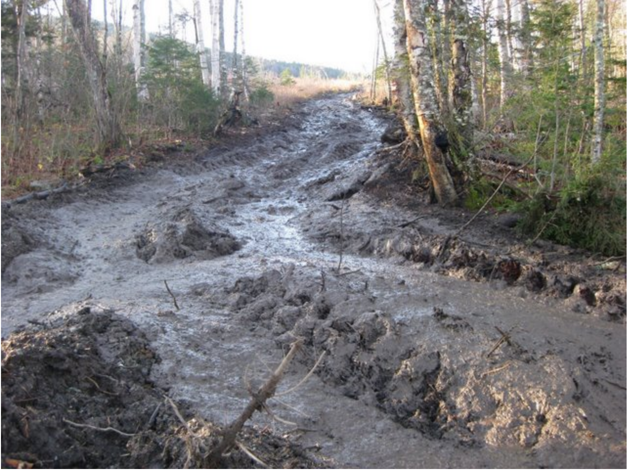
The mud flows are so heavy here it has to pick where it wants to go.....into the breached silt fence or continue down the wheel ruts.
