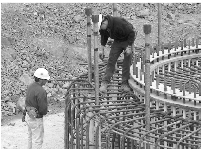
Most of the dozens of site workers are from local Maine contractors. The project has invested over $20 million in Maine.
