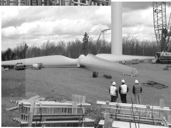
An assembled “rotor” waits to be hoisted up to the top of its tower.
