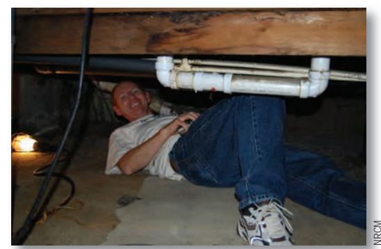
Pete Didisheim insulating pipes under the house to keep them from freezing.
