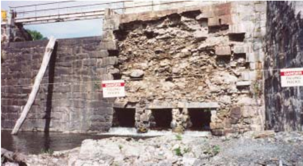
Left: Granite blocks from the Union Gas Dam on Messalonskee Stream in downtown Waterville suddenly collapsed in June 2001. To reduce safety risks, the dam's owner, Florida Power and Light, dismantled a large portion of the dam, allowing the river to run through it.
