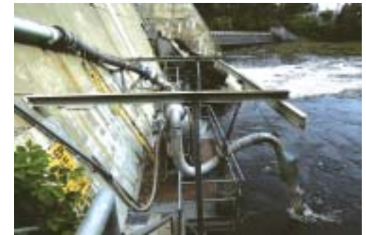
Fish pump at Ft. Halifax Dam on the Sebasticook River.
