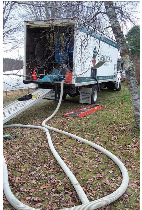
Evergreen Home Performance's cellulose blower truck arrived to install a cellulose "blanket" in the attic and upper crawl spaces.
