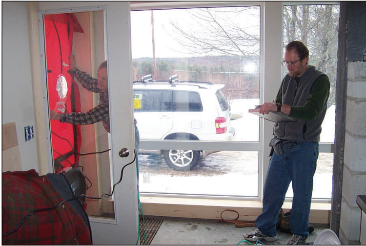
Biff and Charlie of Kennebec Home Performance get ready to measure airflow through the Rectors' house to locate any air leaks.
