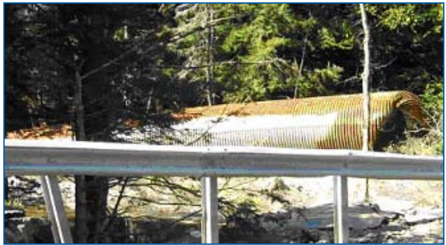
Freeport, Maine road and culvert damage due to insufficient stormwater conveyance capacity at Desert Road
