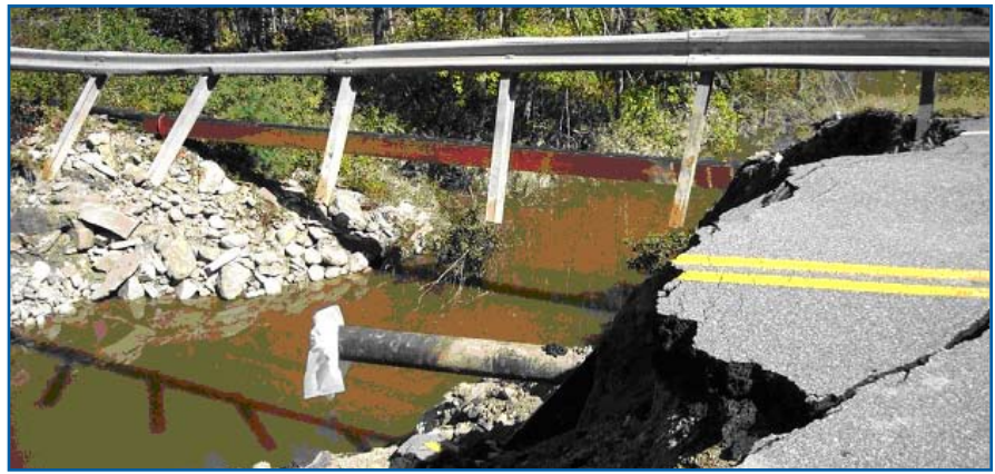
Damaged water main at Desert Road
