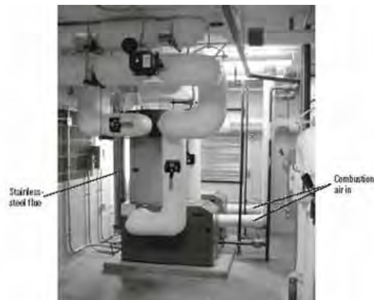
This pair of condensing boilers can be fired at a million Btu's per hour or be throttled back to 67,000 Btu's per hour at steady state efficiencies that range from 92–96%. (Source: Jeff Bowers, Veazey Parrot Durkin & Shoulders.)
