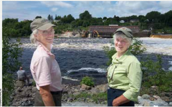
▲ Penobscot River Freed after 200 Years Former NRCM board member Cynthia Hyde (left) and NRCM member Eliza Bailey joined us on the bank of the Penobscot River July 22, 2013, to witness the historic breaching of the Veazie Dam. When removal is complete, the Penobscot will reconnect to the Atlantic Ocean for the first time in nearly 200 years. This is the second major step in the restoration of Maine's largest river, following removal of the Great Works Dam in 2012. NRCM is proud to be a founding member of the Penobscot River Restoration Project.
